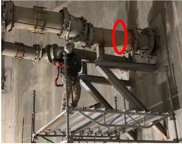
Tank 1 Insertion Valve Location
