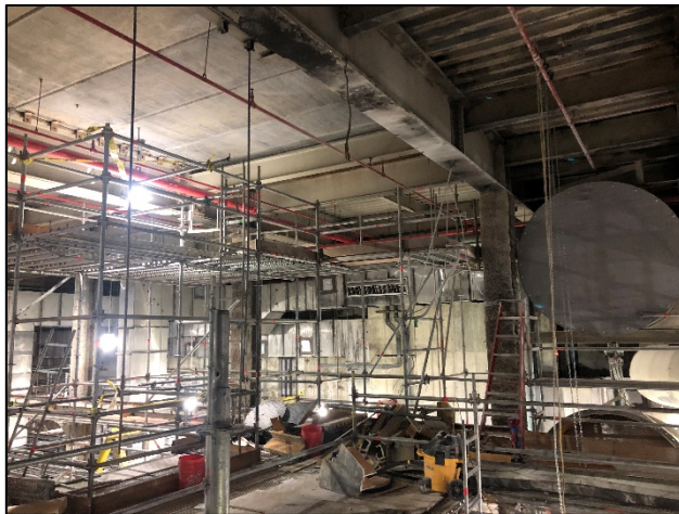
Fire Protection Lines in Odor Control Room
