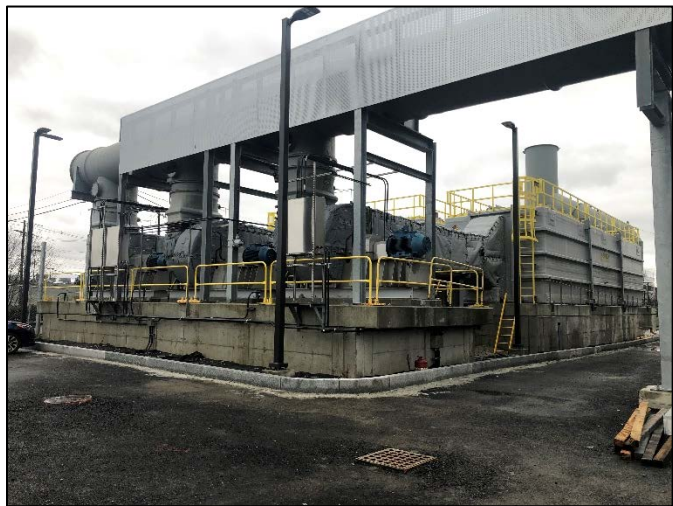
Odor control fan pad with temporary handrails
