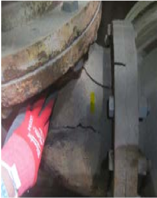
16-Inch Elbow with Crack
