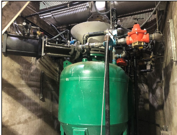
Grit Pod Pit Instrumentation and Controls
