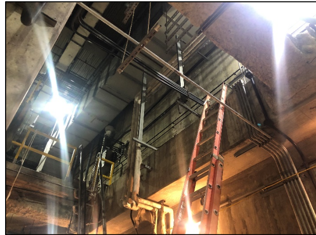
Multiple utilities located within Stair 12
