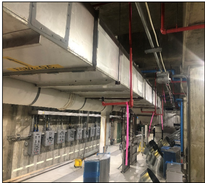
Fire Protection Lines under Ductwork
