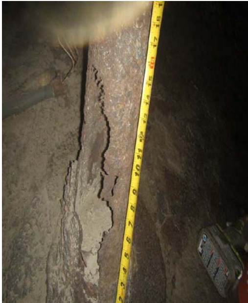
Six-inch Sludge Nozzle with Corroded Hole at Base
