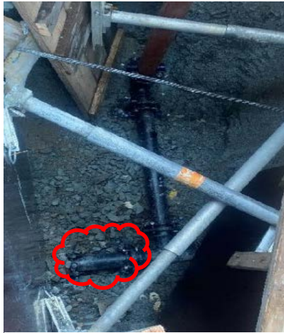
Gravity Thickener 5 Water Connection
